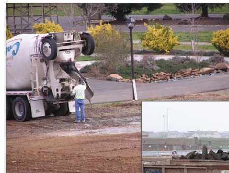
Figure 1. Chute washwater being dumped on the ground
