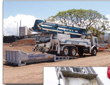
Figure 14. Pump truck using the ramp to wash out into a roll-off bin
